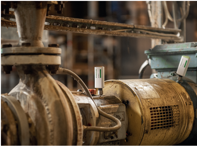
Condition monitoring solution Paper mill: OPTIME CM does well in engine monitoring
