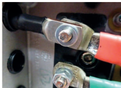
65 U V W power cable and washer
